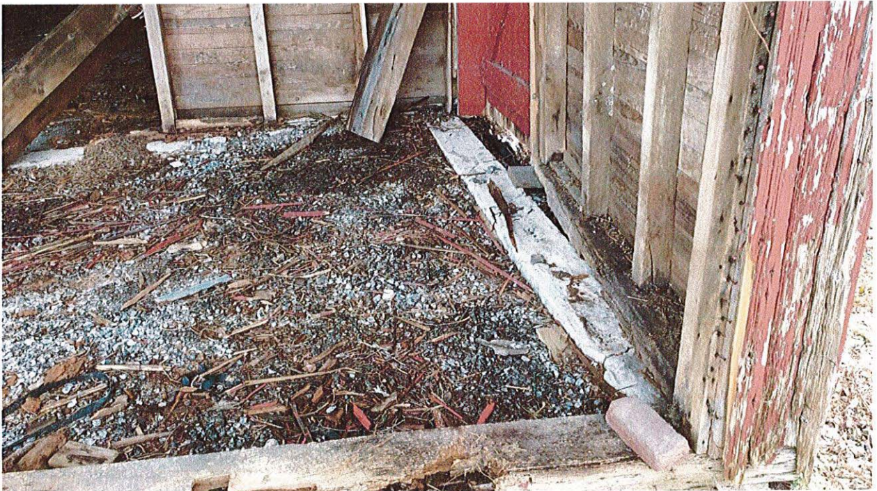
Photo 8. Barn sill plate shifted off foundation southwest corner.
