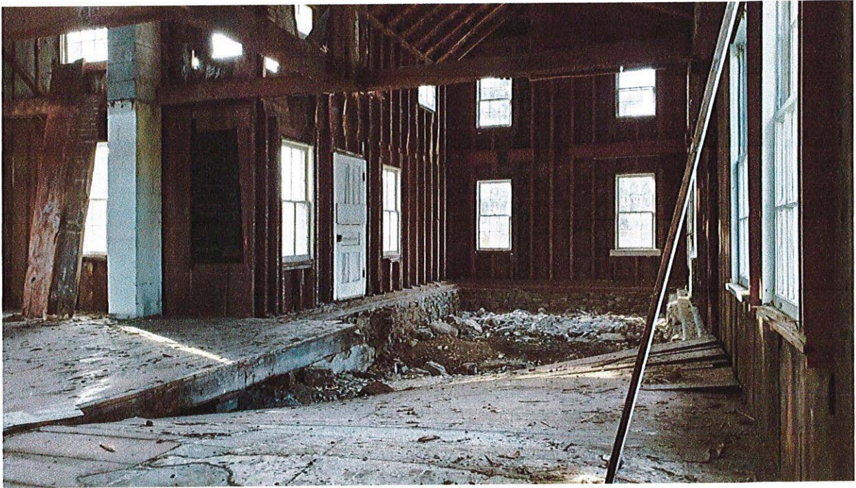
Photo 3. Gutted interior with collapsed floor, middle portion and south end of house.
