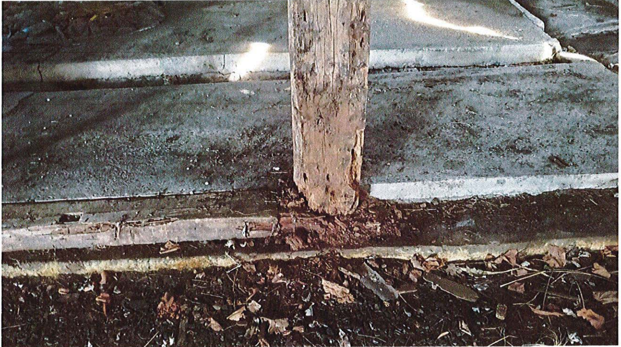
Photo 7. Interior barn wood column, rotted at base (typical).
