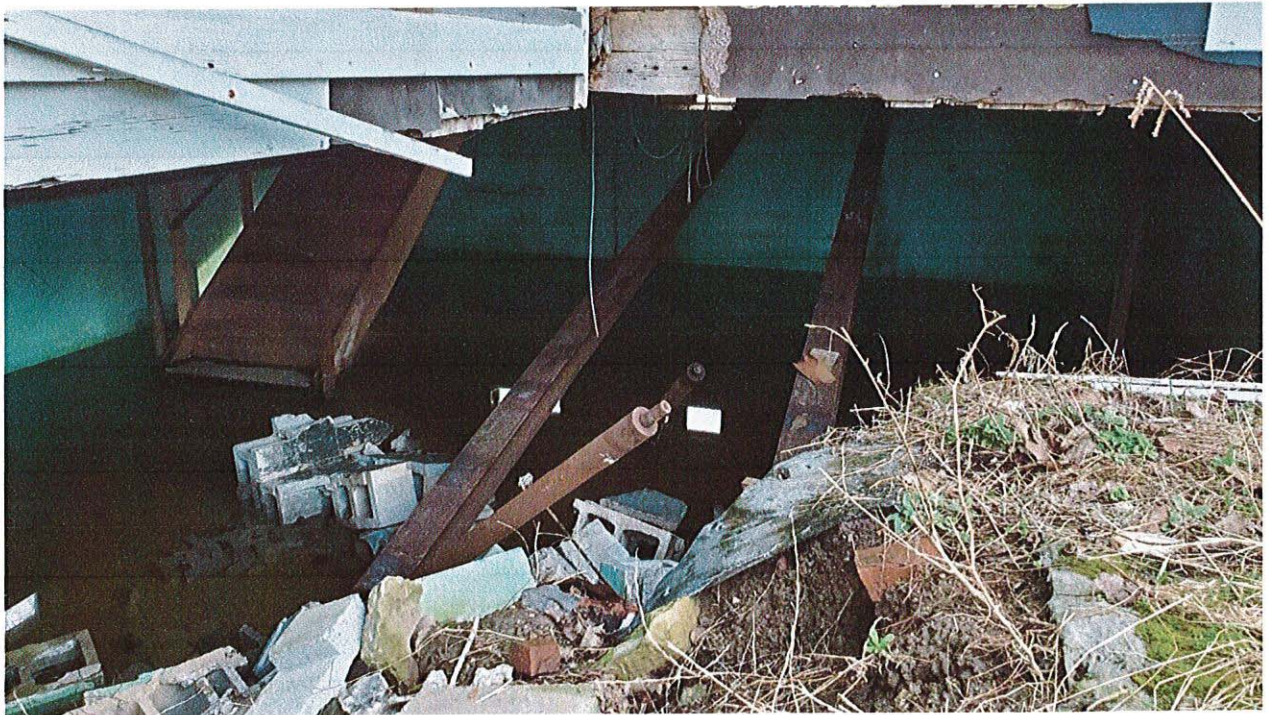
Photo 2. Collapsed foundation and steel beams on west side of house.
