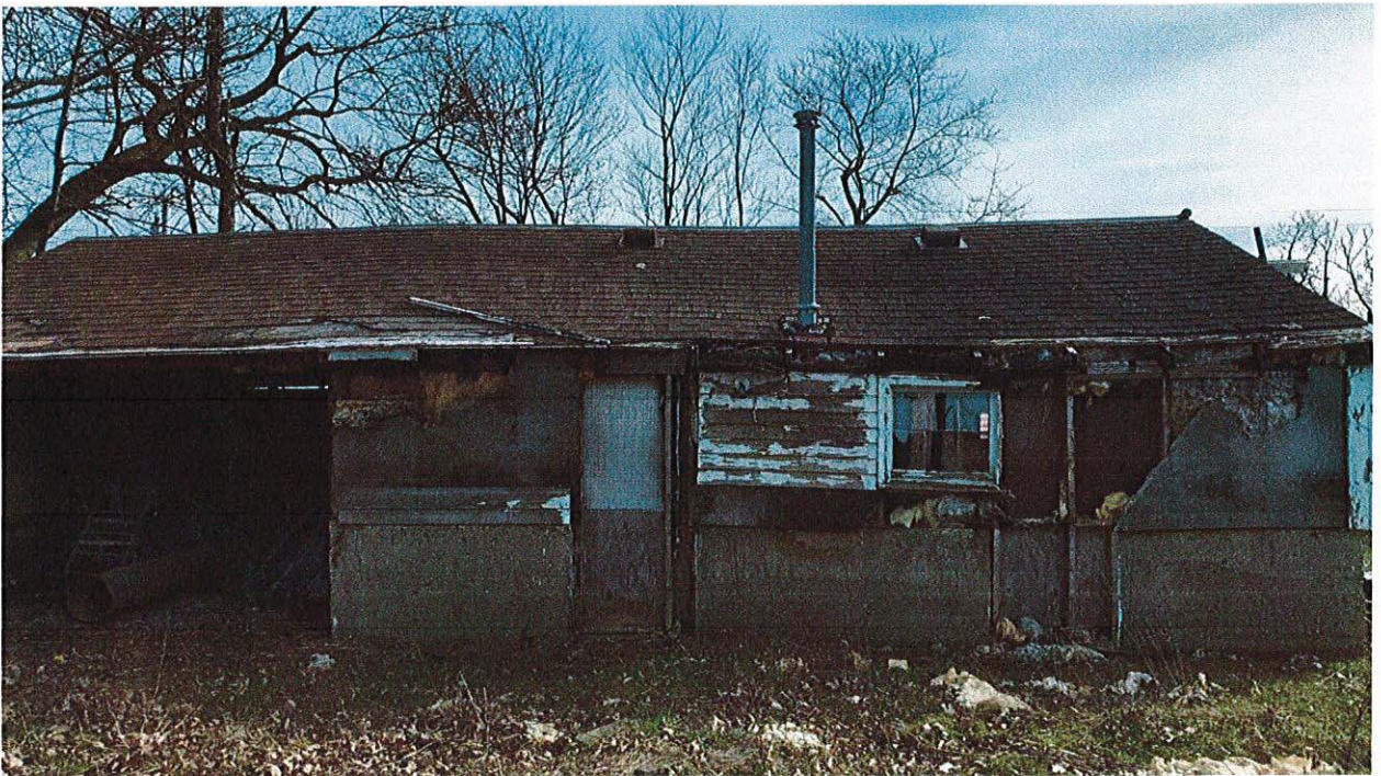
Photo 10. West Side of shed/garage with missing siding, gutters and fascia. Note foundation settlement.
