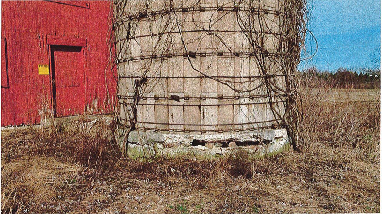
Photo 9. Deteriorated silo foundation.
