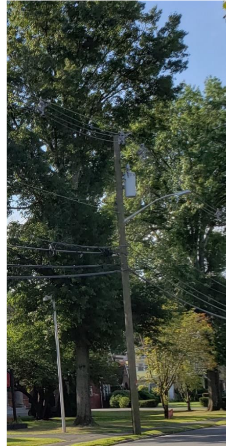
Photograph 3. Representative photo of tree inventory identified tree conflicts with the higher voltage primary transmission lines, above the transformer.
