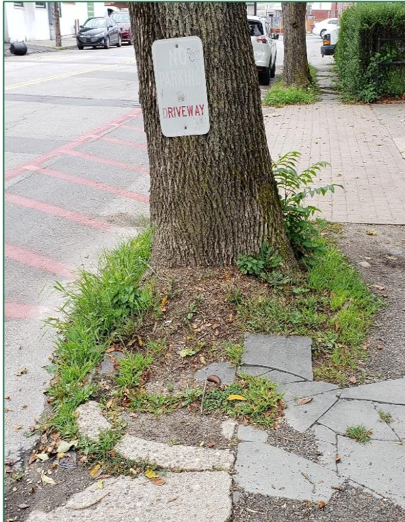
Photograph 4. Potential sidewalk damage may occur– choose the right tree for the right place.
