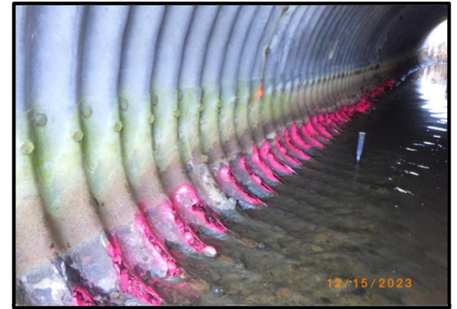
Existing Photo: Section loss holes in structure, looking southwest in Span 1.
